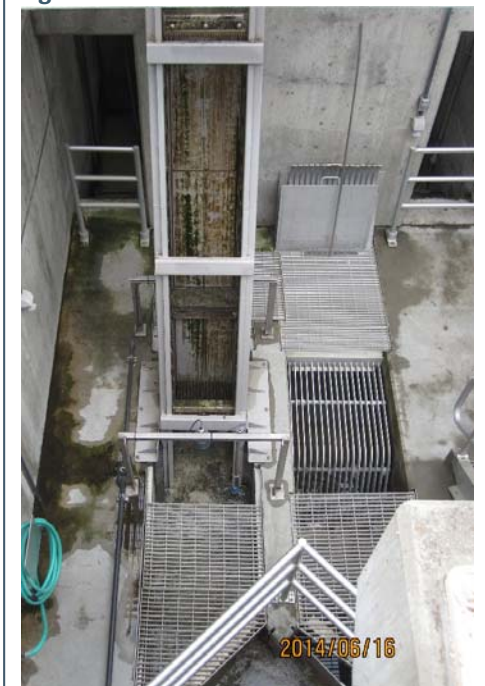
Figure 8-6: Headworks Screen Channels
