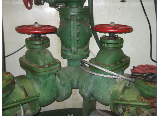
Figure 7-6: Highway 1 Lift Station Dry pit
