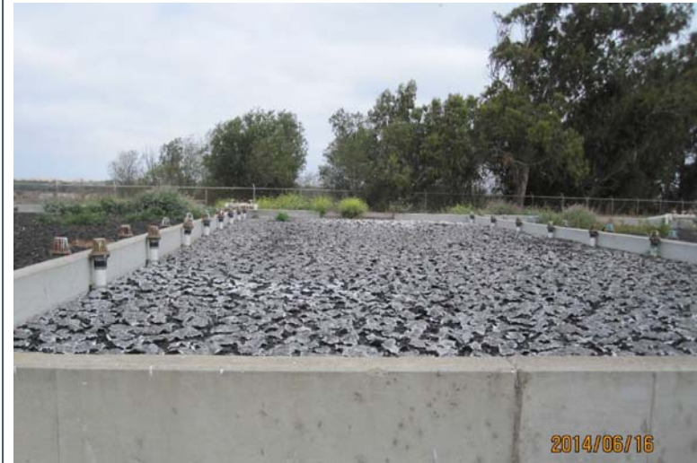
Figure 8-11: Sludge Drying Beds
