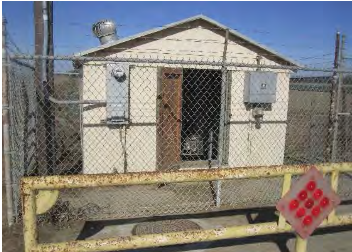
Figure 9-3 Pioneer Street Lift Station
