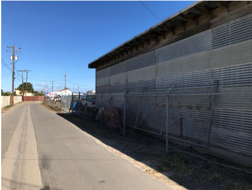
View from South to North (Fence structure is in generally good shape.)
