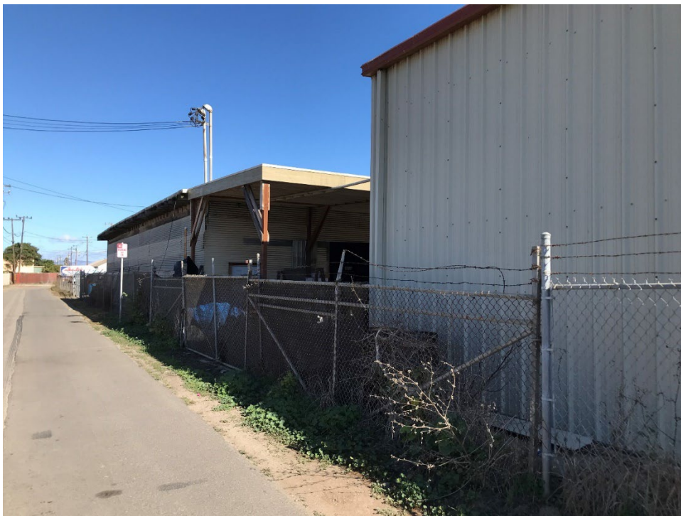
View from South to North (Fence structure is in generally good shape. The fence barbwire is damaged approximately 60 feet from the Southwest corner of the lot. The area of barbwire needing repair is approximately 44 feet in length.)
