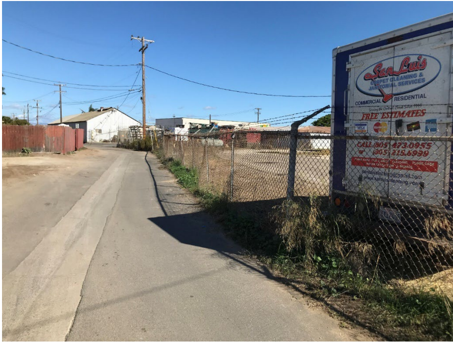
View from South to North (Fence structure is in generally good shape. Repair of fence bindings, straightening of fence poles, tightening of the fence, and weed abatement required.)
