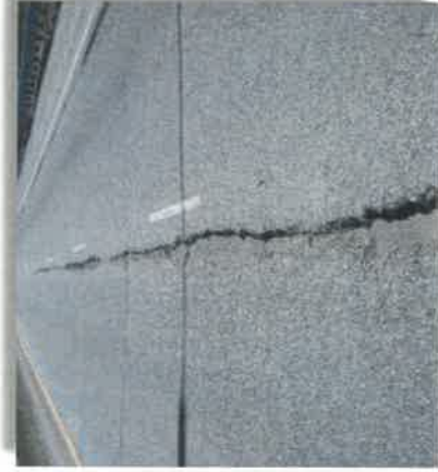
Transverse or Longitudinal Cracking
