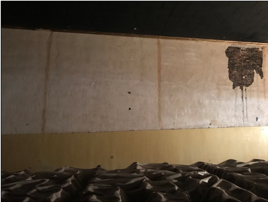
Plate 26. South wall of theater showing evidence of electrical fire.
