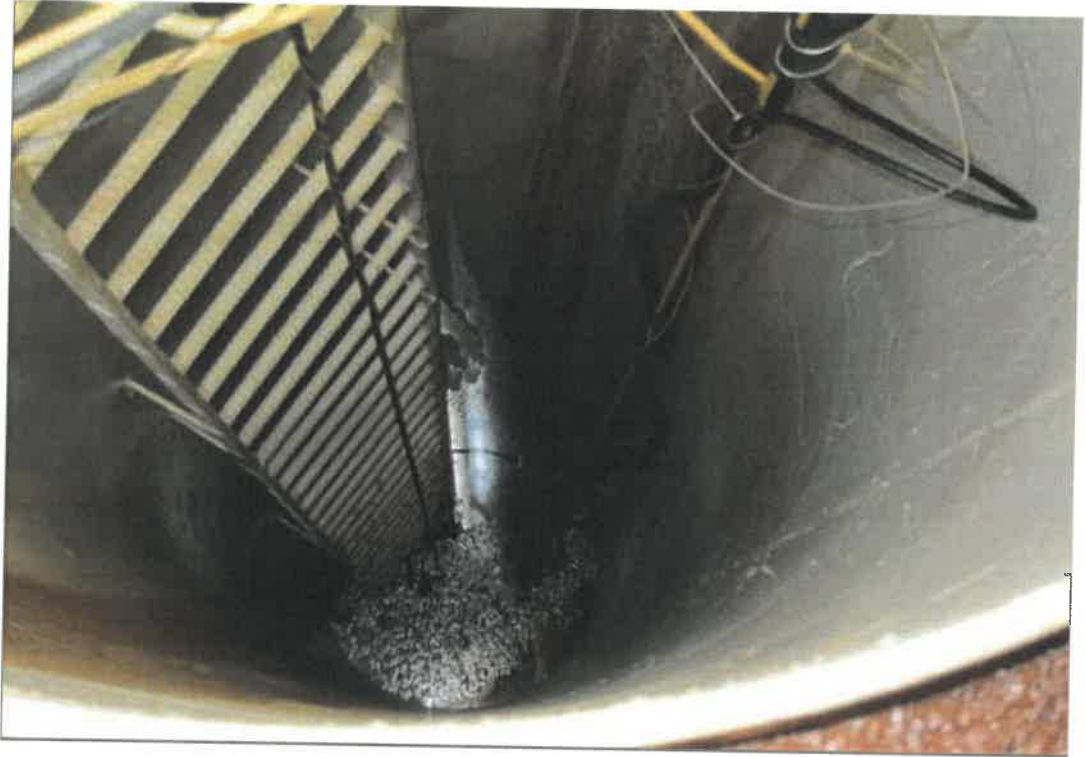
Interior of the riser pipe. The pipe surfaces appeared to be free of significant corrosion.
