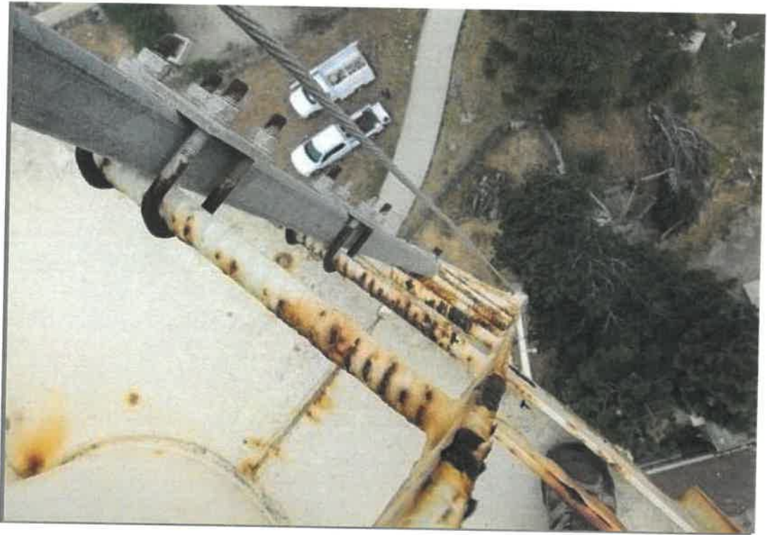
This view from the top of the exterior ladder shows the overall condition. Significant corrosion and metal loss are present.
