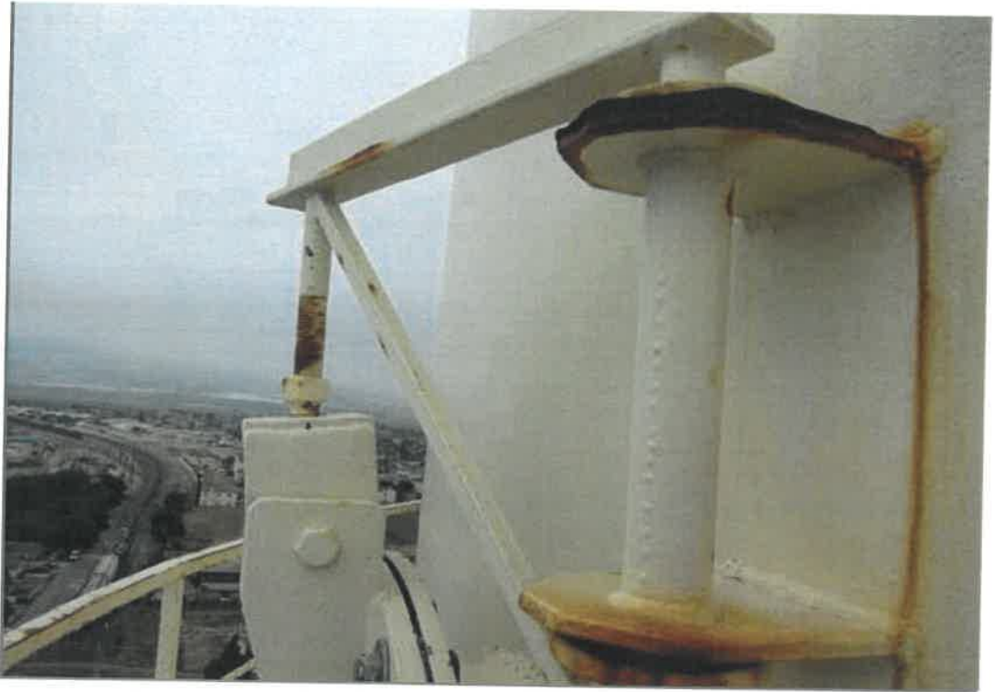
Significant corrosion is present on the exterior of the shell manway hinge and davit.
