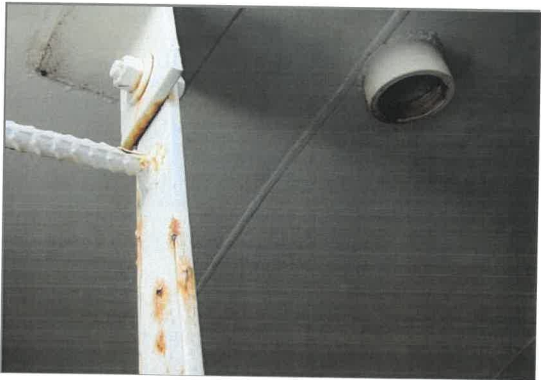
Upper end of the interior ladder and a roof mounted coupling. Rust is visible on both.
