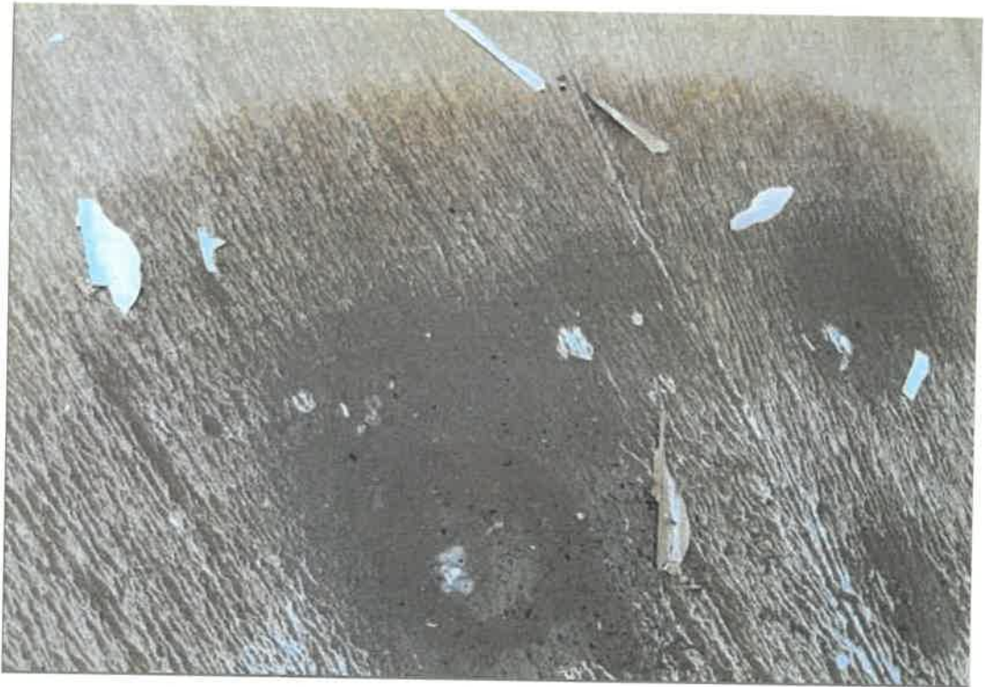
This photo shows the typical condition of the bottom. Some paint chips are visible and they appear to be from the interior ladder.
