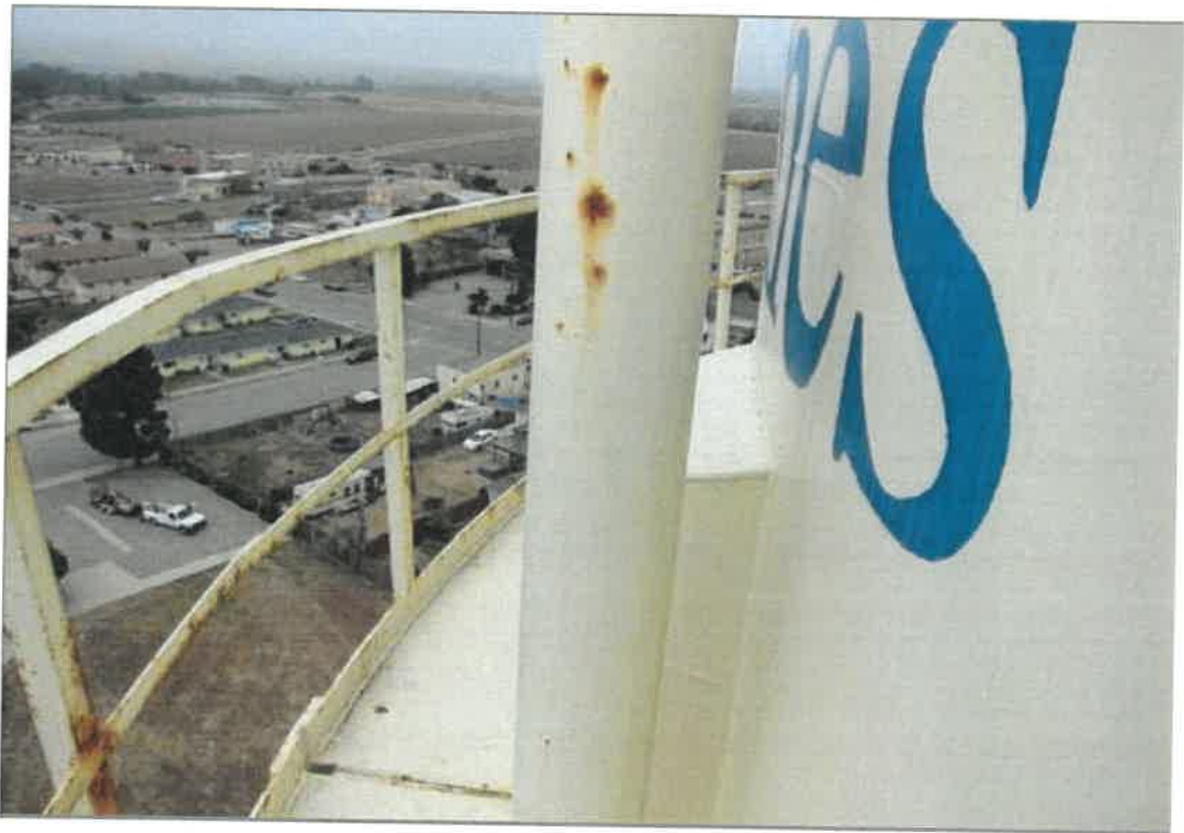
Overflow pipe with corrosion on the exterior.
