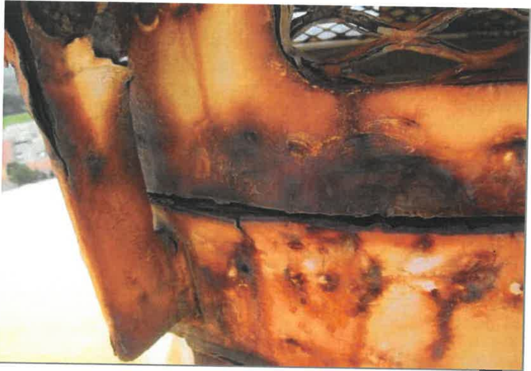
This view shows some of the serious corrosion on exterior of the roof vent.
