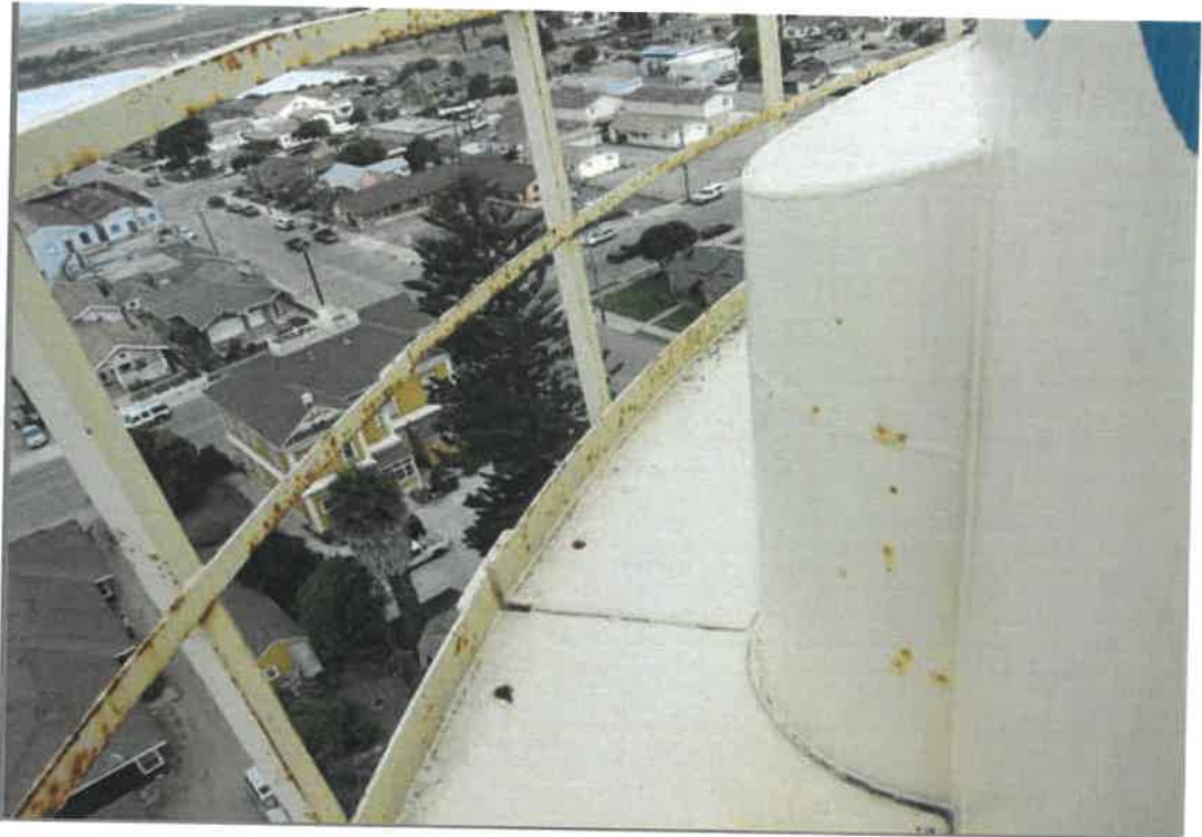
Exterior view showing the typical condition of the columns at the tank connection. Corrosion is present.
