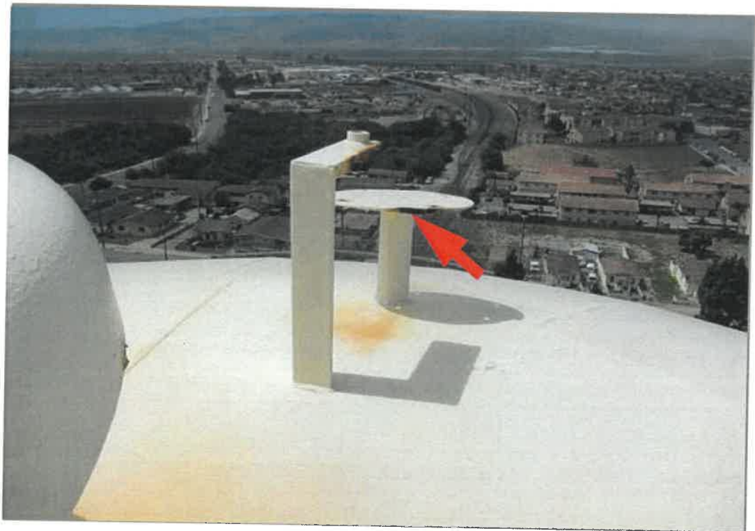
Roof mounted appurtenance brackets with significant corrosion.
