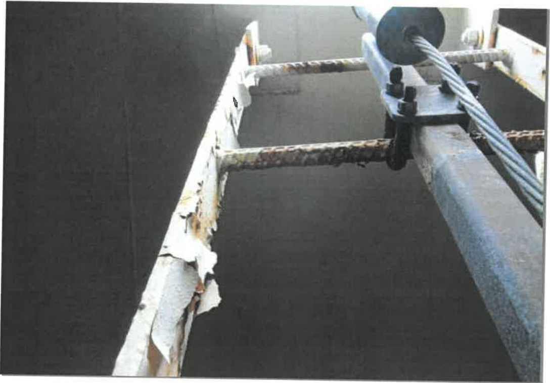
Interior ladder near the top. The final coat of coating on the ladder is peeling away on most surfaces. Rungs and climber safety device have serious corrosion.
