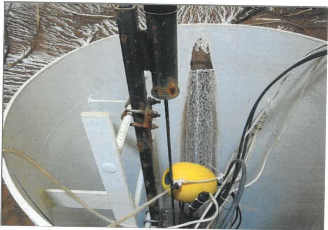
Top of the riser pipe. The climber's safety device has some significant corrosion.
