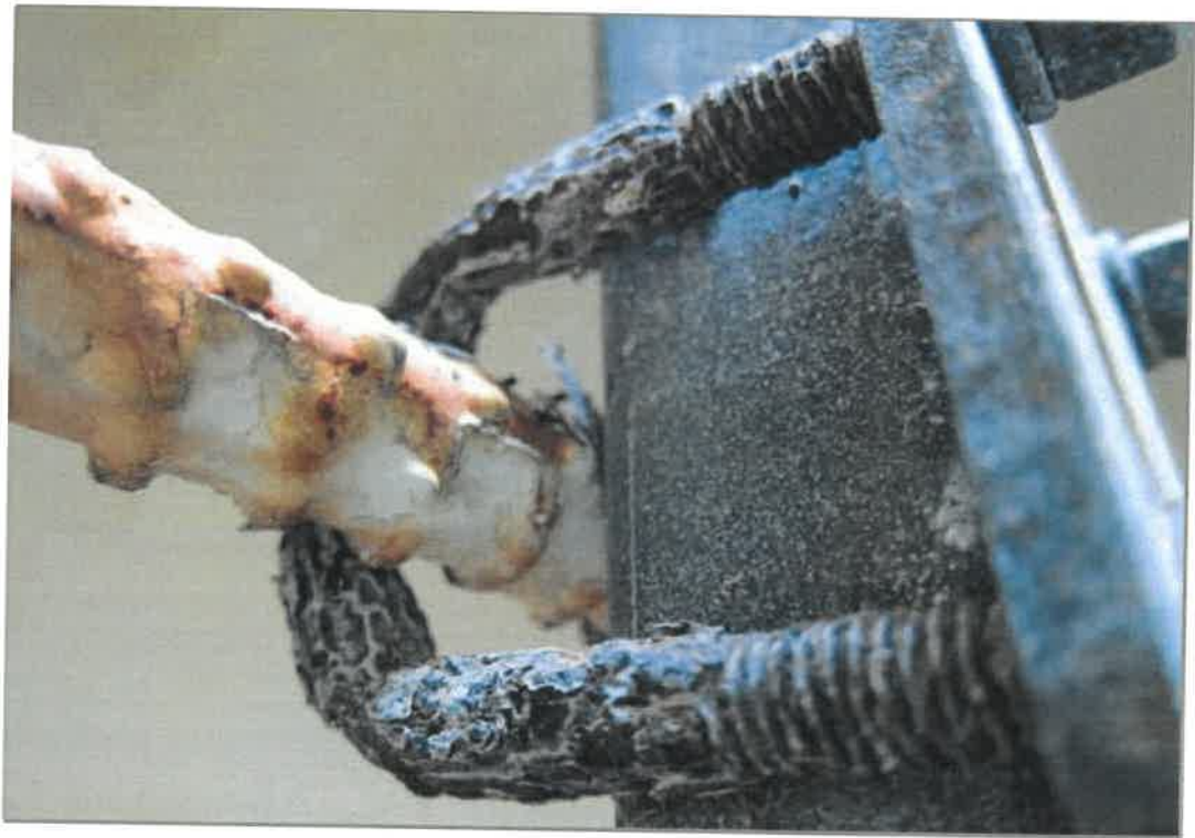
Close view of interior ladder and climber safety device at the top of the ladder with significant corrosion.
