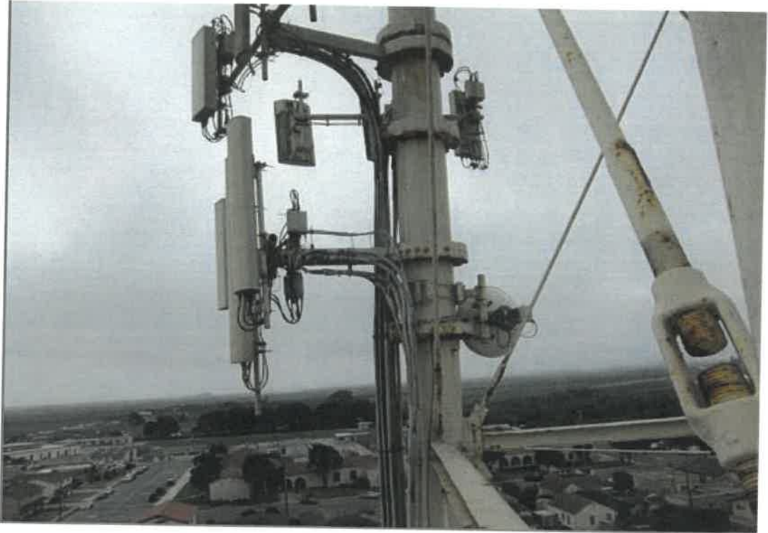
Various antennae and conduit on the upper column. Supporting structure and brackets appear to have similar scattered corrosion as other exterior surfaces.
