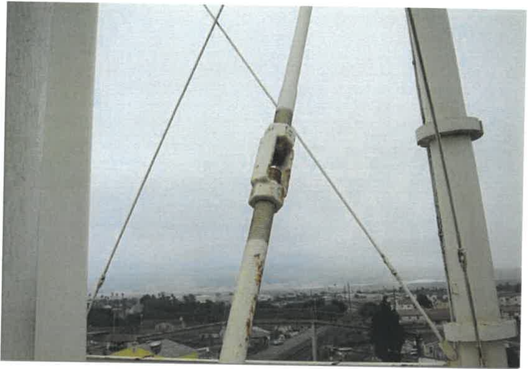
Exterior view showing the typical condition of the turnbuckle on wind bracing Minor corrosion is scattered.
