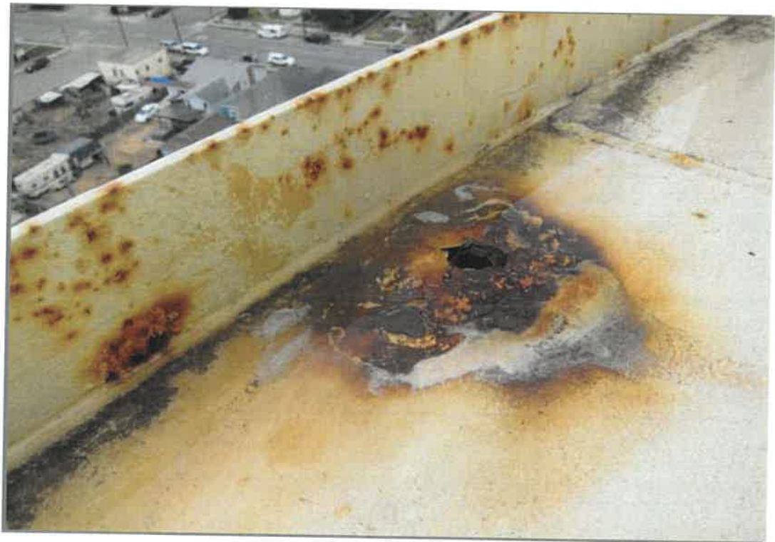
Significant corrosion and metal loss (rust grade D) are present on the balcony. Ponding appears to be accelerating coating failure and corrosion in this area.
