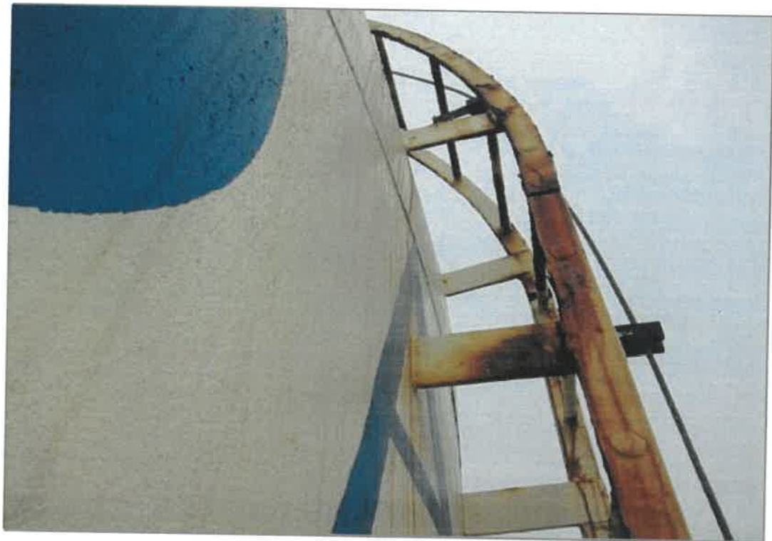
This view of the tank shell mounted portion of the exterior shell ladder shows the poor condition due to corrosion (rust grade C)
