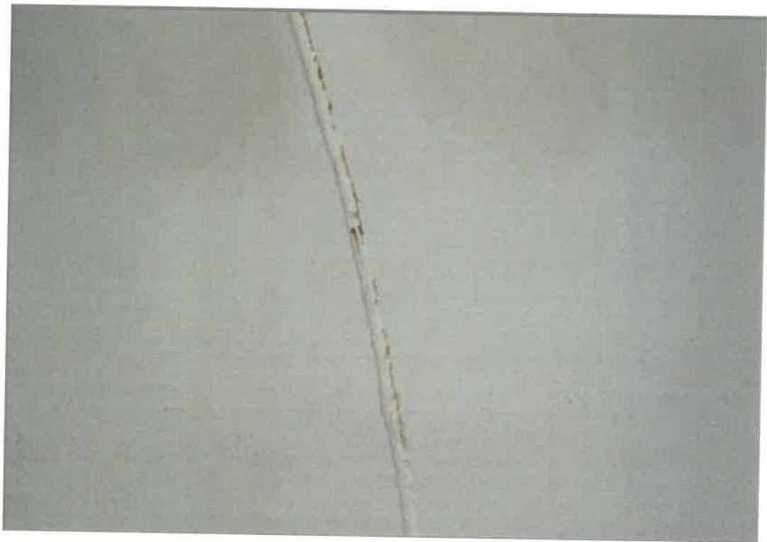
This view of a weld on the northern side of the interior of the dome roof shows the worst corrosion on the interior roof.
