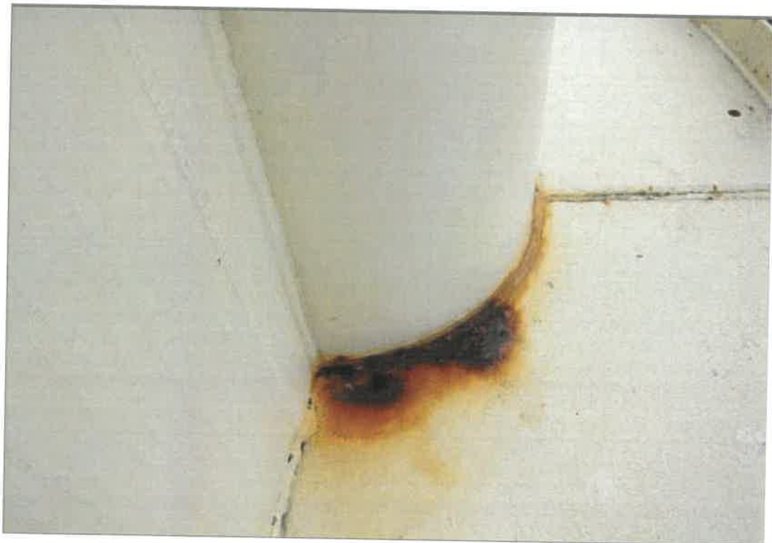
This view shows significant corrosion (rust grade C-D) on the column at the balcony walkway. Ponding is accelerating corrosion here.
