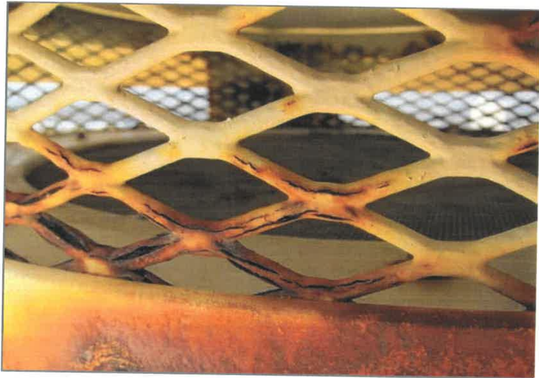
Corrosion is present on the exterior but the stainless steel screen on the interior appears to be intact and bug proof.
