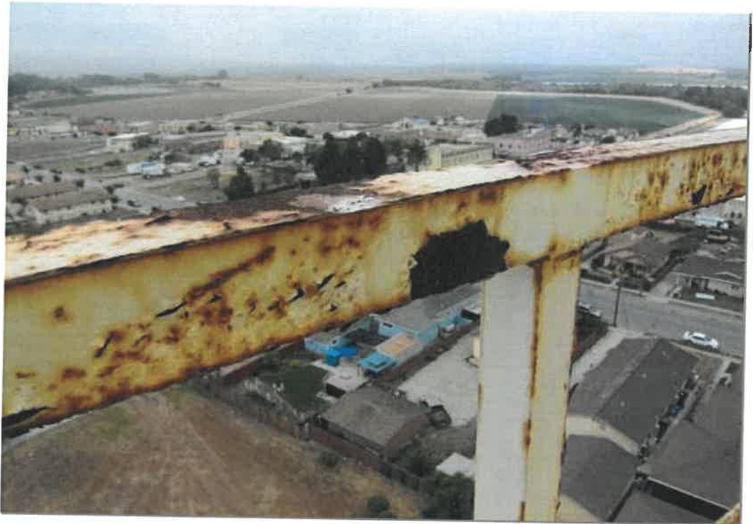
This view of the guardrail shows the significant corrosion on the railing.
