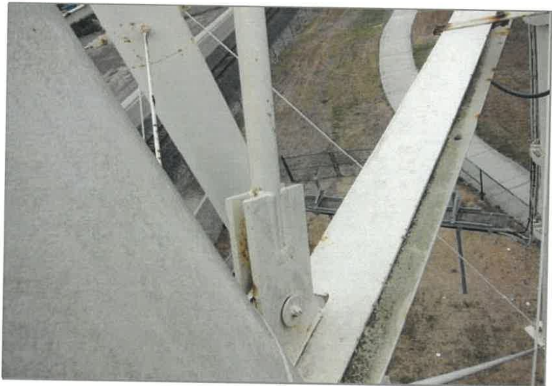
A column, lower strut and windage rod (brace) is shown here. Minor scattered corrosion (rust grade B) is visible
