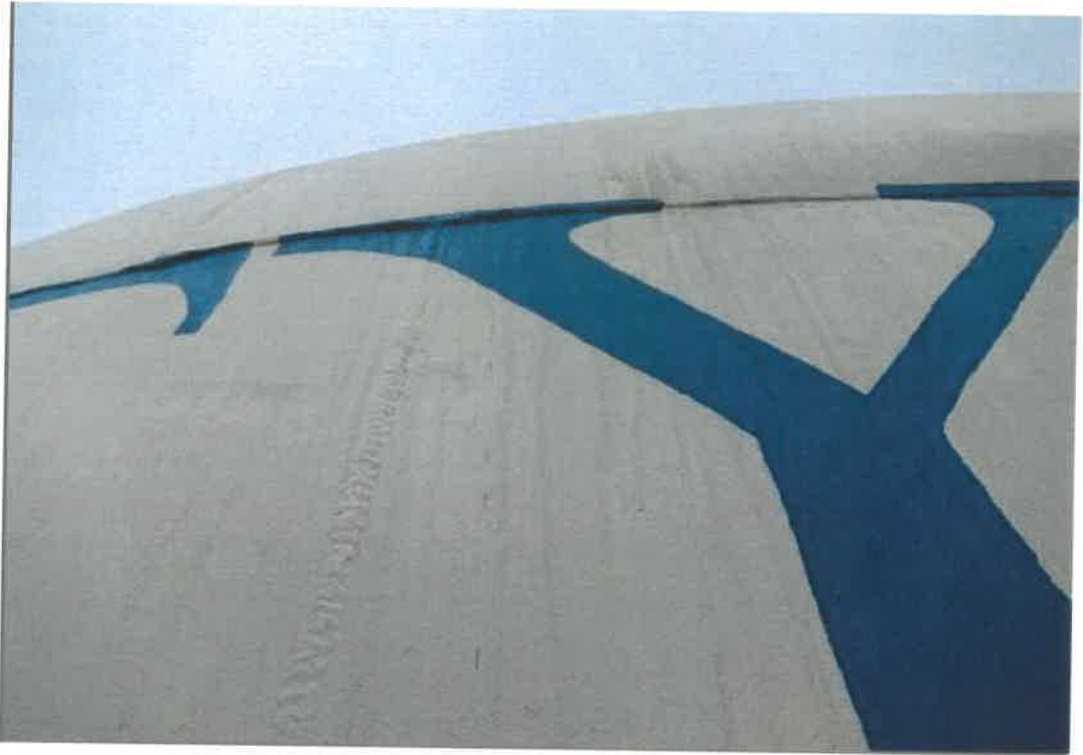
This view represents the typical conditions on the upper shell and shell to roof joint. The upper shell is in good condition with 8 minor corrosion points noted.
