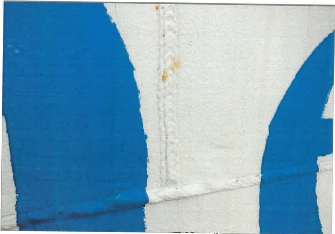
A vertical and horizontal shell weld junction are shown here. The condition shown is typical of the upper exterior shell with some minor corrosion present.
