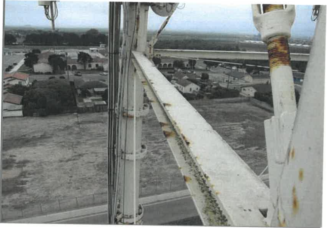
This view of upper strut on the north side shows another example of what appears to be the typical corrosion conditions on the exterior structure.
