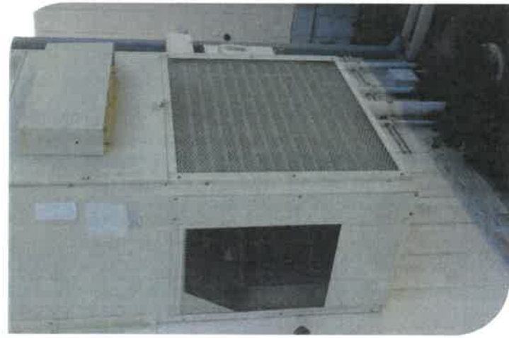
Old HVAC systems need to be replaced with energy efficient models
