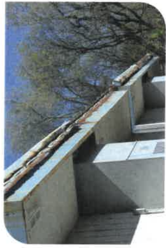
Leaky and damaged roofs and ceilings must be repaired
