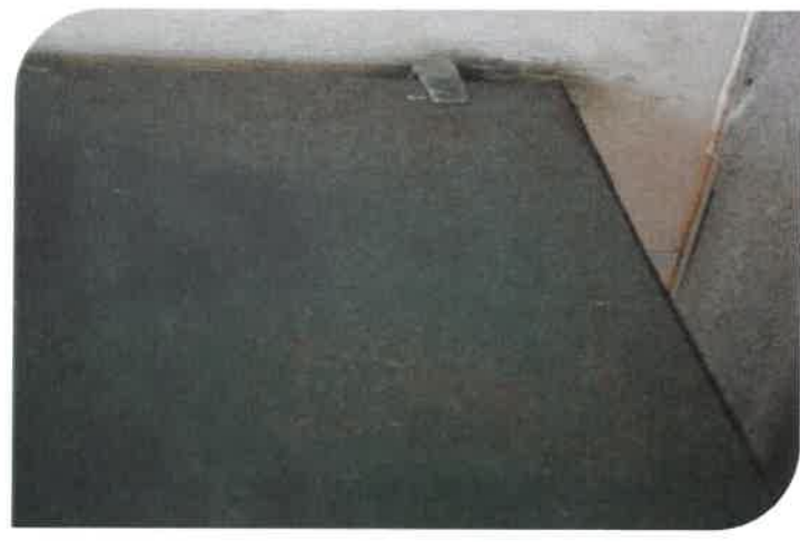
Significant renovation/modernization is needed
