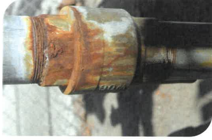
Deteriorating plumbing systems need to be replaced
