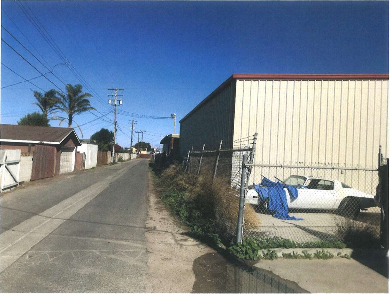
View from South to North (Southwest corner of the property at 333 Guadalupe St. Fence structure is in generally good shape. The gate and the initial 15 feet of the fence have leaned inward. Straightening of poles and Weed Abatement on the fence line is required.)
