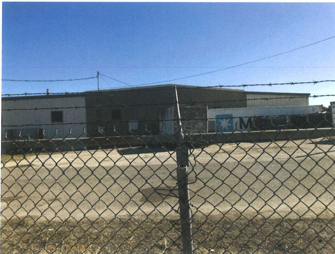
View from West to East (Fence structure is in generally good shape. Repair of fence bindings, straightening of fence poles, and remounting of pole bracket is required.)
