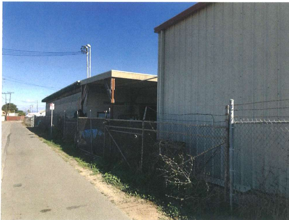
View from South to North (Fence structure is in generally good shape. The fence barbwire is damaged approximately 60 feet from the Southwest corner of the lot. The area of barbwire needing repair is approximately 44 feet in length.)
