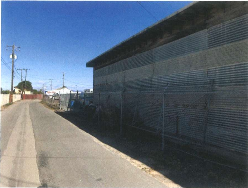
View from South to North (Fence structure is in generally good shape.)
