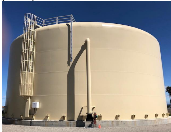
City of Guadalupe New Obispo Tank #2 Storage Tank
