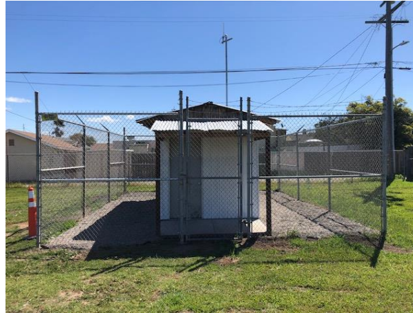
City of Guadalupe New Tognazzini Well 2A
