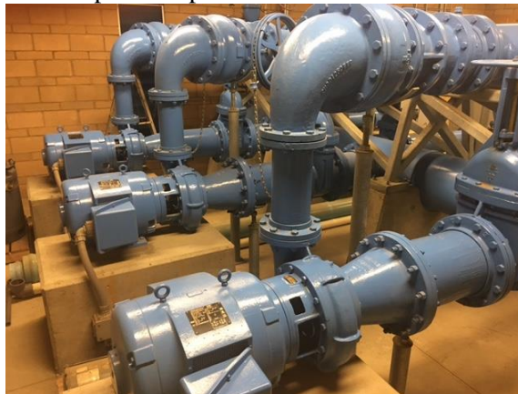
City of Guadalupe Fire Flow Pumps- Boosting Station
