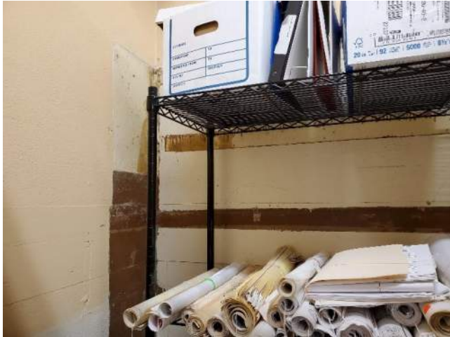
Figure 24: Storage Racks - No Anchorage 01.
