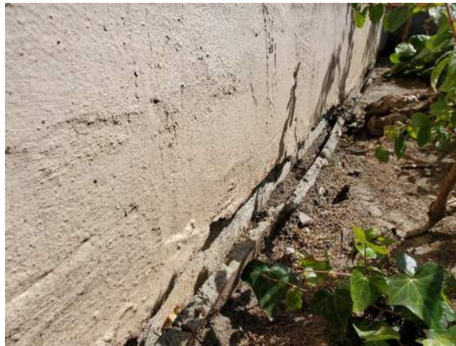
Figure 57: Exterior Grading and Stucco at Foundation 02.
