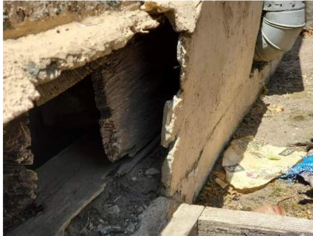
Figure 37: Structural Deterioration at Crawl Space Vents 02.
