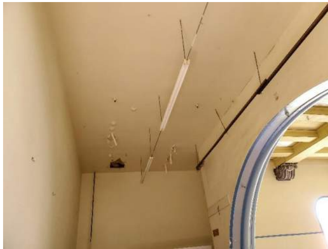
Figure 17: Water Damage at Ceiling above Stage.
