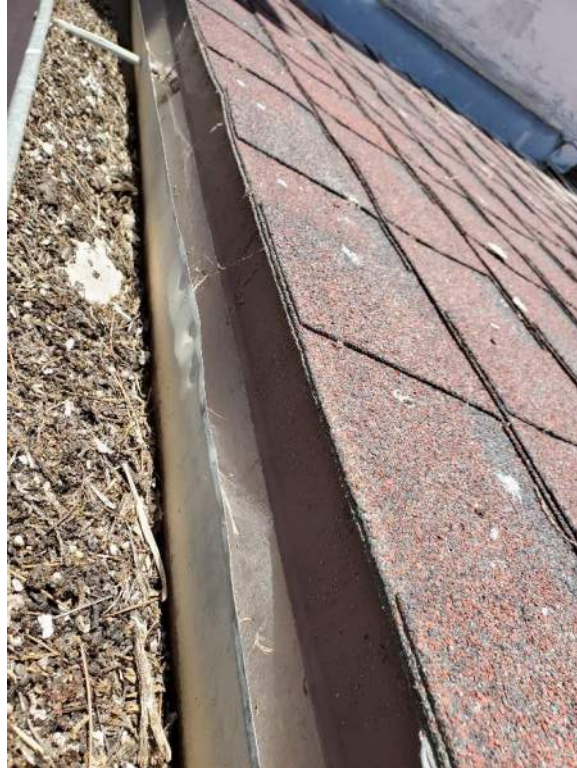
Figure 52: Existing Gutters Require Maintenance.
