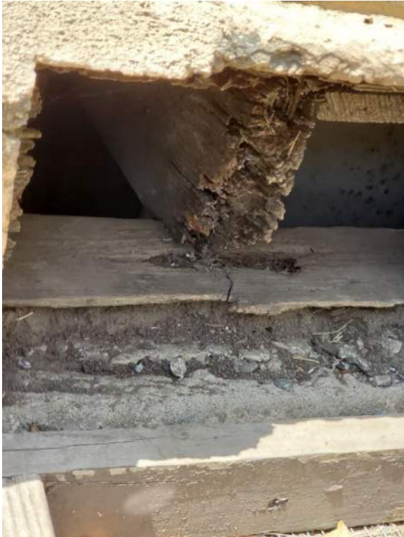
Figure 36: Structural Deterioration at Crawl Space Vents 01.
