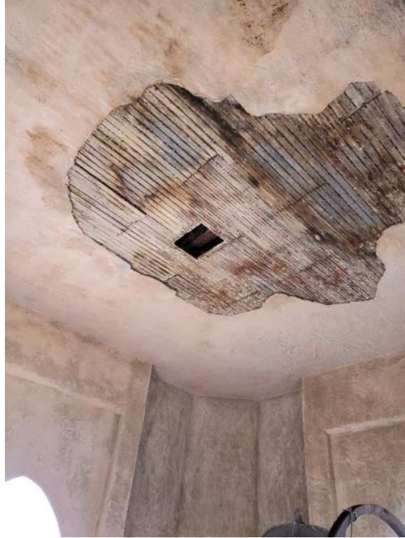
Figure 48: Interior Plaster Ceiling Needs Repair at Bell Tower.
