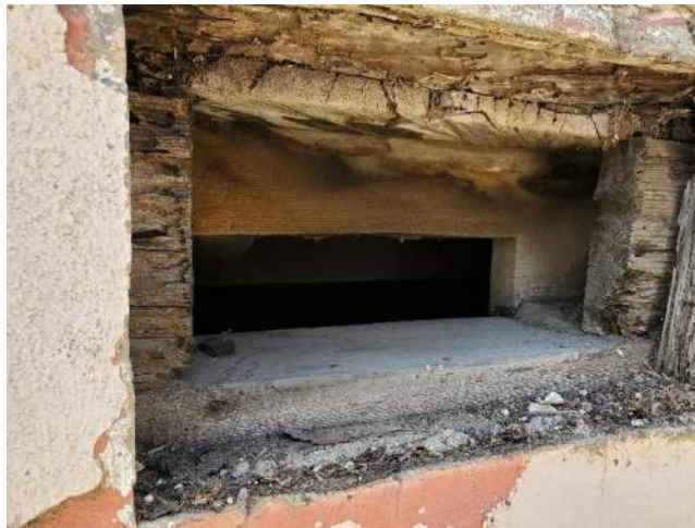
Figure 38: Structural Deterioration at Crawl Space Vents 03.
