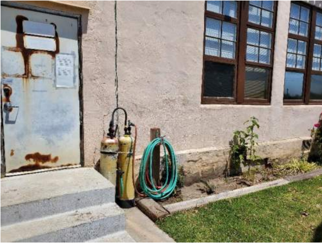
Figure 20: Exterior Wall at Fire Department 02.
