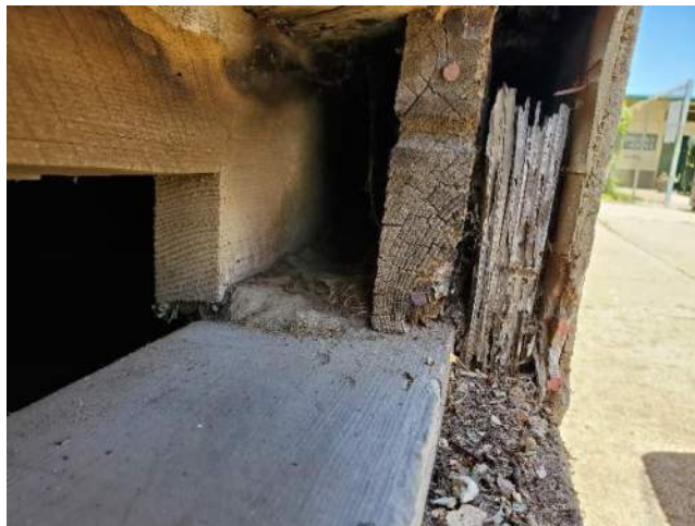
Figure 39: Structural Deterioration at Crawl Space Vents 04.
