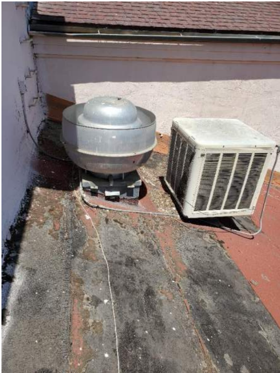
Figure 45: Mechanical Equipment at Roof.
