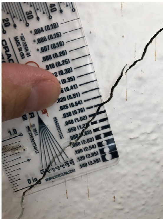
Figure 4: Observed cracking of interior finishes
