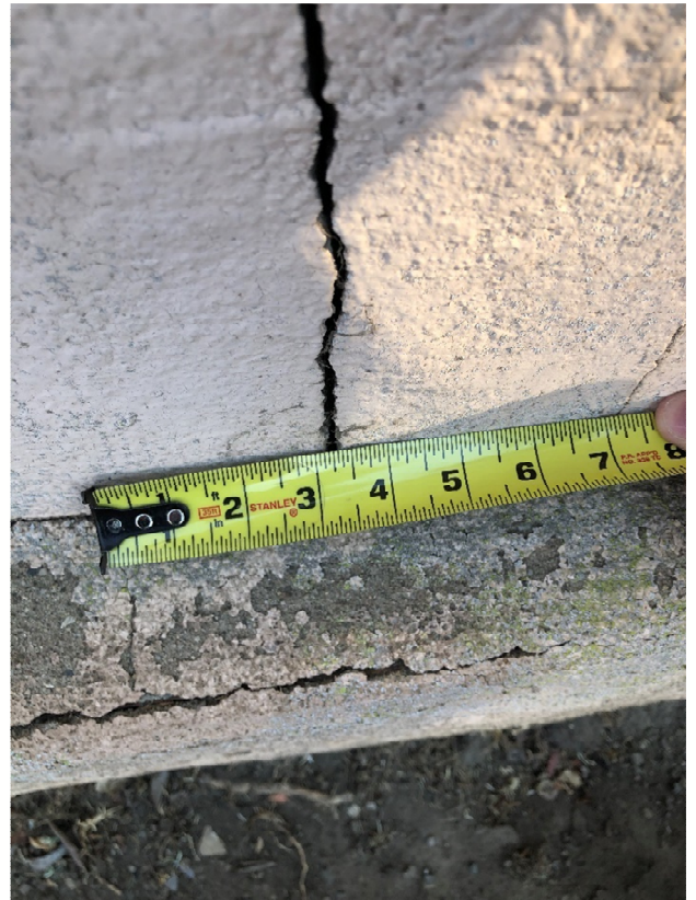
Figure 7: Cracks in exterior plaster likely leading to water intrusion into the wood floor framing system
