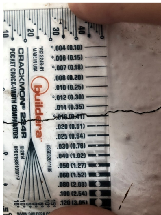
Figure 5: Observed cracking of interior finishes
