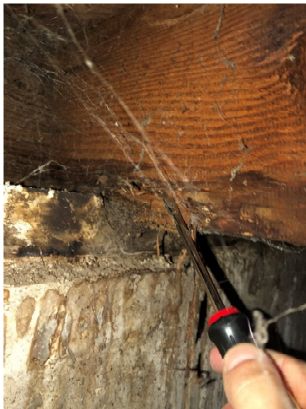
Figure 2: Observed damage to joist and sill plate
