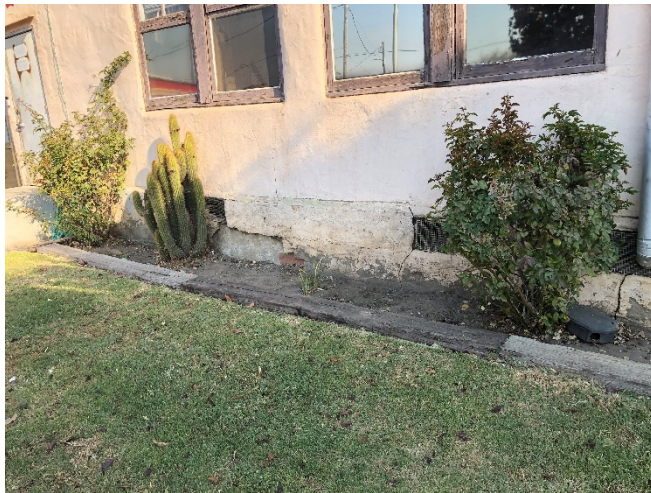
Figure 6: Exterior Wall of the Fire Department. Location of vents are consistent with the location of crushed of sill plates
