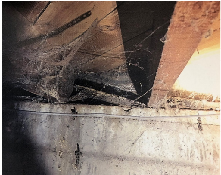
Figure 3: Observed crushing of sill plates from joists J10 and beyond
