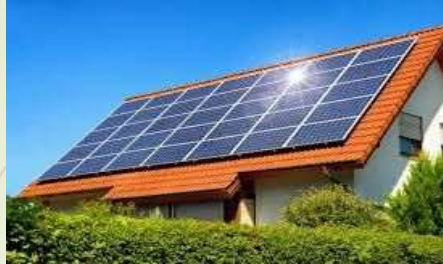
Solar panel installations
